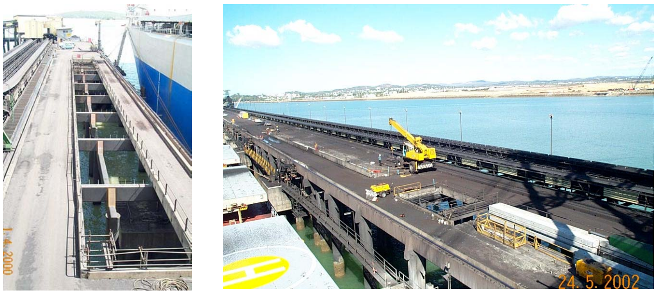
Figure 7. The new infill supports in place, and closing the gap in the deck.
